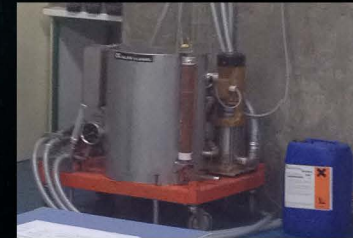
View of part of the cooling system where the primary circuit transfers heat to the secondary circuit
