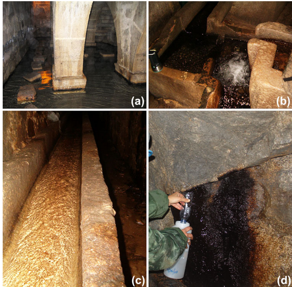
Fig. 2 Some aspects of the spring galleries catchworks: a Arca d'Água masonry reservoir (ca. XVI century); b junction of Paranhos and Salgueiros spring waters; c granitic gutter pipe; d seepage from an open sub-horizontal discontinuity
